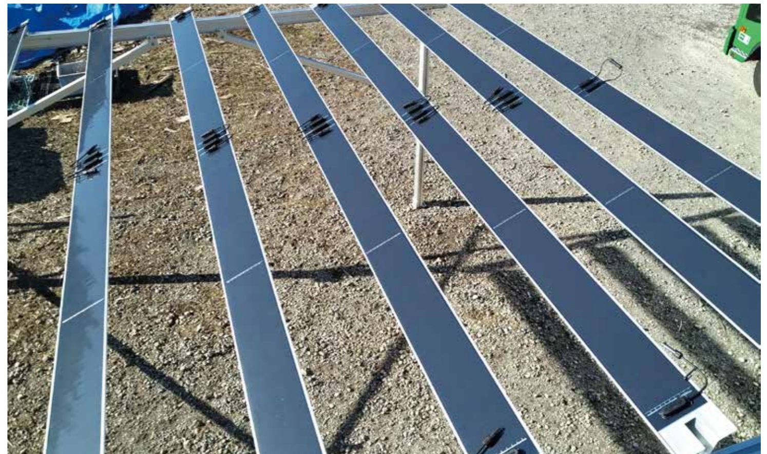
Temporary installation of the prototype that arrived. The ease of installation was almost as intended, and with this reality, development has made great strides, and we are one step closer to completion.
